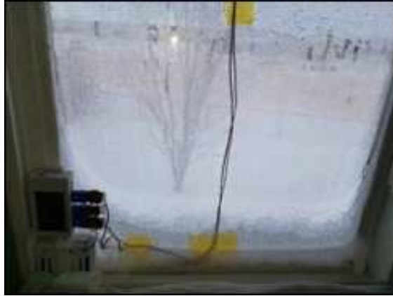
Condensation and ice buildup on existing double-pane
